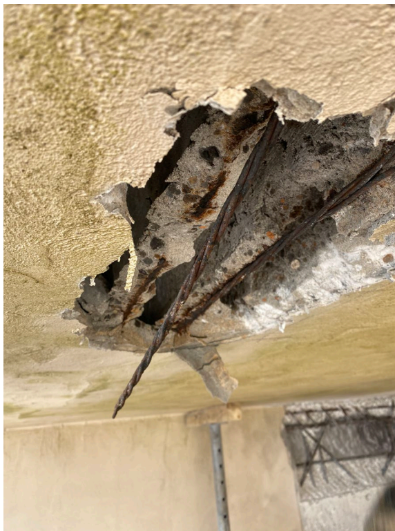
Picture 5: Broken tendons in ceiling of slab below Unit 108
